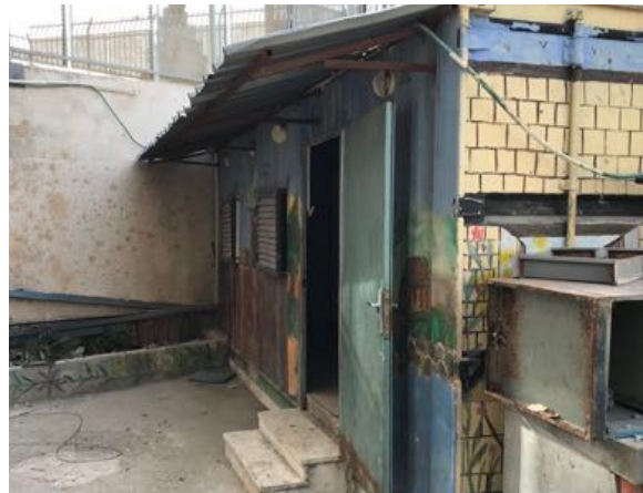
This ramshackle facility was the only toilet for the 350 boys of the school
